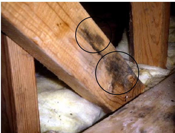
Circled areas show mold fungi growing on wooden beams.
