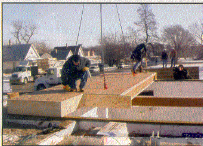
Workers set the deck for the 2,000 sq. ft. home in Omaha, NE.
