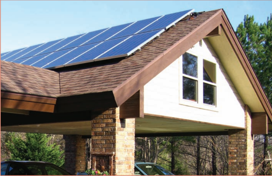
The complete PV array on the pavilion behind the house helps Stitt sell solar. "You've got to have something for people to see," he says.
