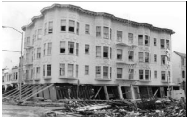
San Francisco, CA, 10/89 Loma Prieta earthquake. Rubble from a collapsed Marina District apartment building litters one lot while nearby, a building is shored up. FEMA News Photo
