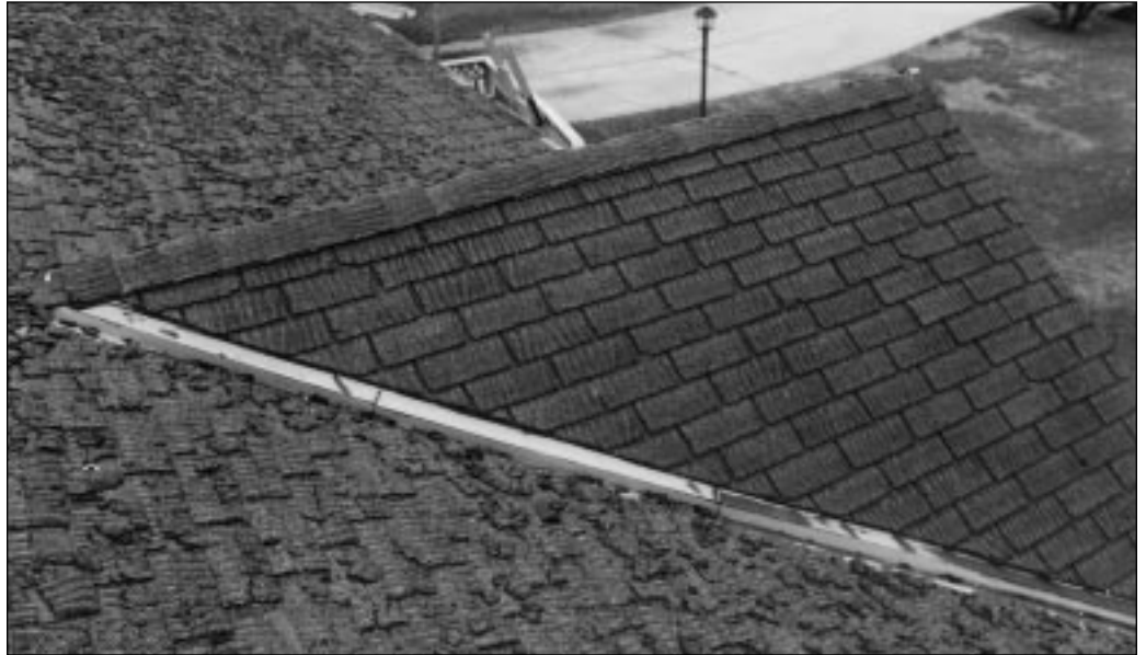
Hail resistant roofing can significantly reduce the damage shown.
