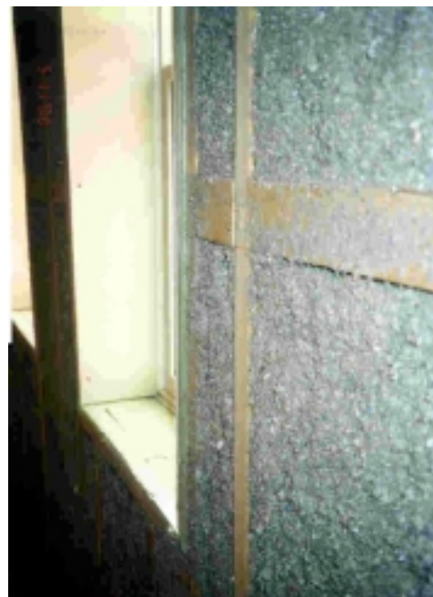
Existing walls were furred-out to provide a cavity for the blown-in cellulose insulation.
