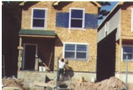
Sealing around windows. Note sheathing is not interrupted by rim joist.
