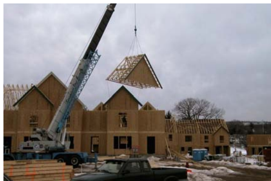
Large truss assemblies were lifted into position and secured with hurricane clips and truss floater clips, which allow for differential expansion
