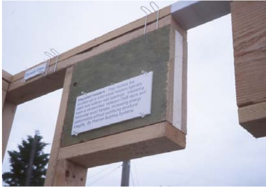
Drywall clips/stops (at top plate) and insulated header
